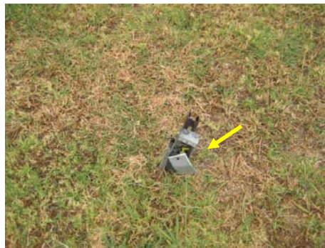
Figure 12 Missing cover plate-front parkway
