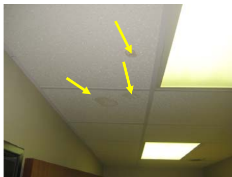
Figure 26 Water stain-Center storage closet
