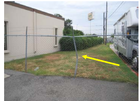
Figure 19 Damaged fence-West side rear
