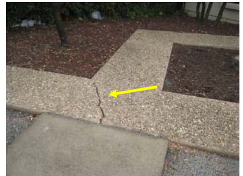
Figure 11 Cracked sidewalk example-front
