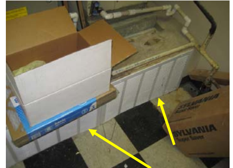
Figure 23 Return air in Closet
