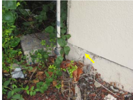
Figure 16 Corner crack- SW corner
