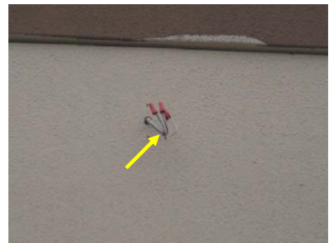
Figure 9 Exposed wires/missing light front ext.
