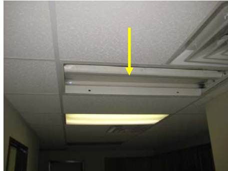
Figure 22 Missing light diffuser-example
