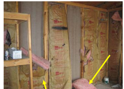
Figure 21 fallen insulation-rear storage building
