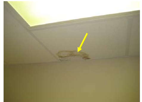
Figure 25 Water stain-Center storage closet
