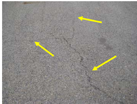
Figure 10 Common cracks in asphalt parking area
