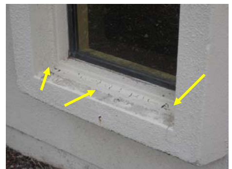
Figure 15 Minor flaking paint-example
