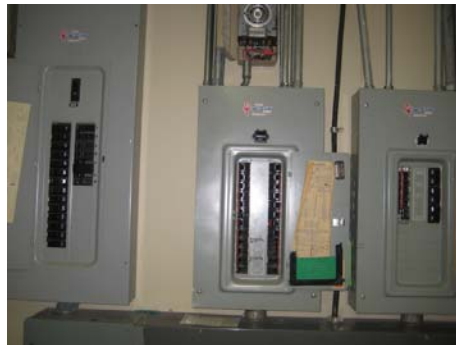
Figure 24 Panel boxes (L-R) 200 amp, 150 amp, 150 amp
