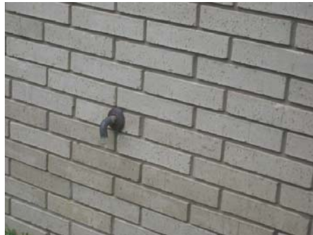
Figure 9 Water heater Temperature pressure relief line-too high-West side ext.
