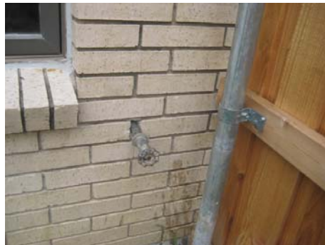
Figure 1 Loose hose connection-East
