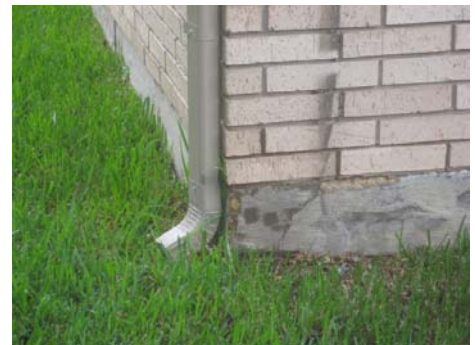
Figure 4 Missing gutter downspout splashblock
