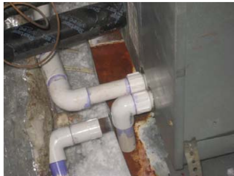
Figure 19 East AC unit-pan holds water
