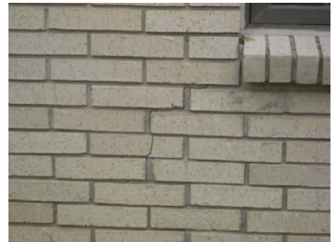
Figure 2 Cracked mortar/brick-East side
