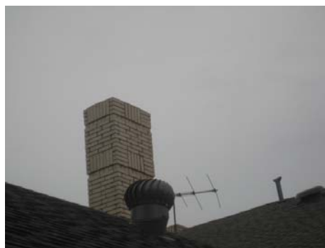
Figure 5 Missing chimney cap--rear
