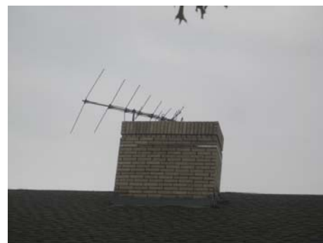
Figure 14 Missing fireplace chimney cap-front
