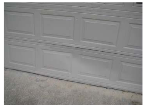
Figure 6 Damaged garage door
