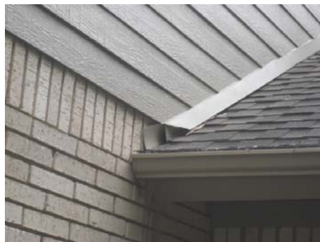
Figure 11 Missing sidewall flashing-West side
