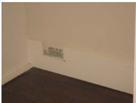
Figure 15 Missing refrigerator receptacle cover
