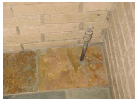
Figure 12 Missing hose connection handle
