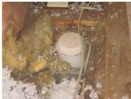
Figure 21 Recessed lights touching insulation
